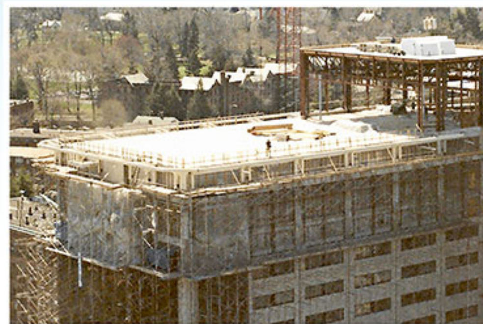
Construction on the helipad atop Hartford Hospital began in 1989. The completion of the helipad and hangar cleared the path for other construction projects on campus.
